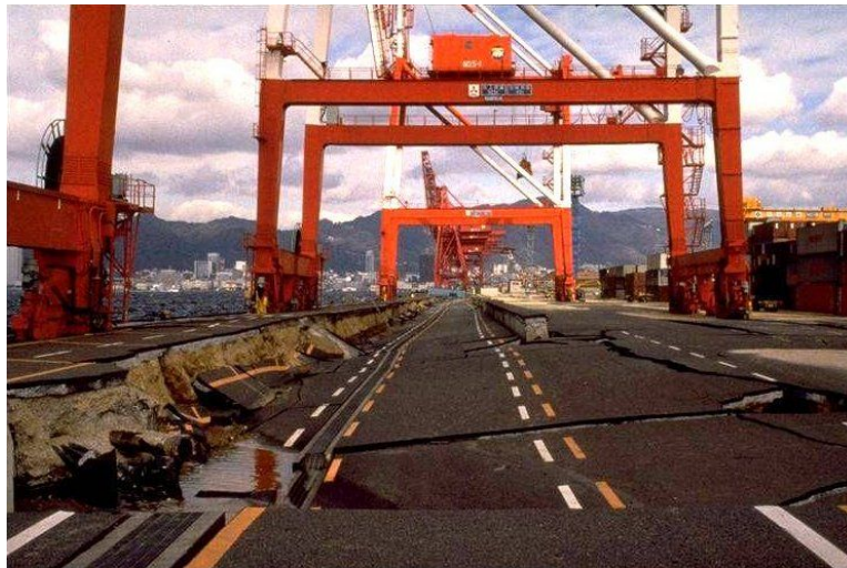
Figure 1. Damage to the rear-line region of the dock caisson induced by the 1995 Great Hanshin-Awaji Earthquake, Kobe Port (Kobe Geotechnical Collection, 2019).
